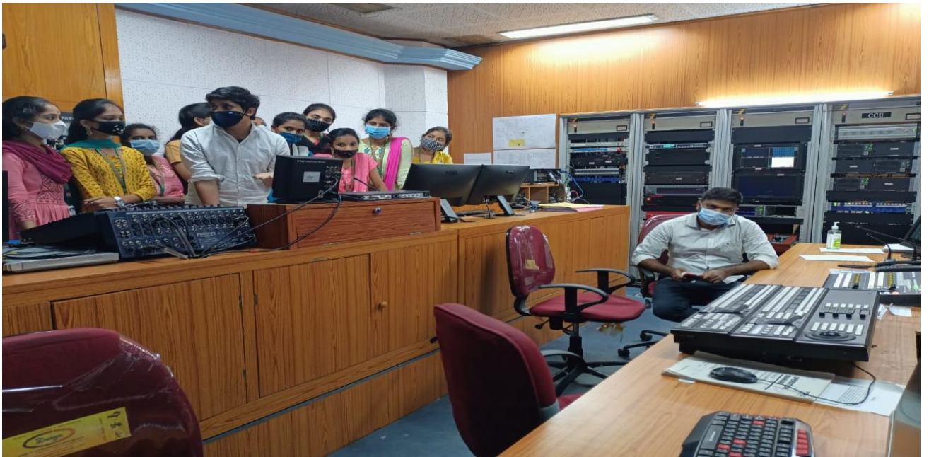
Photos: Doordarshan Kendra Vijayawada Video and Audio Processing Units, High Power Earth station Transmitter unit
